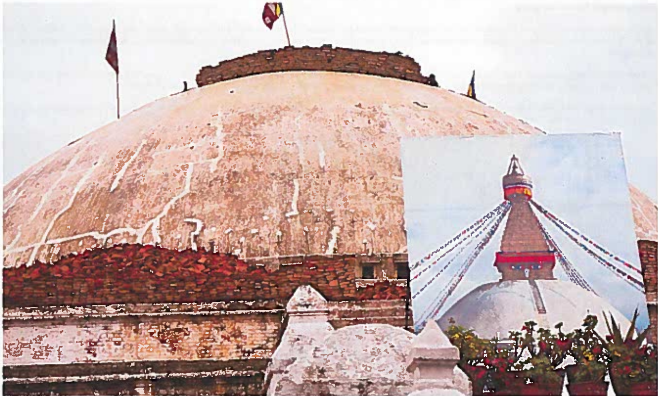
Before and after: In Kathmandu, Nepal, Boudhnath's great stupa is undergoing reconstruction to fix structural damage caused by the April 2015 earthquake Photo Credit: Jeff Greenwald
